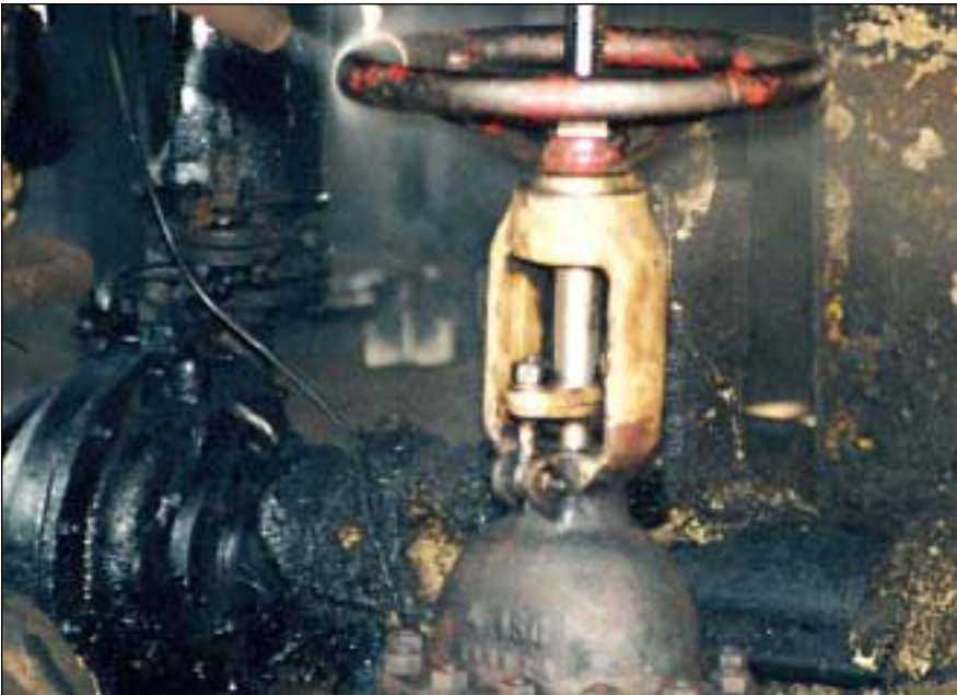
Cleaning nearly complete with valve still in place. Note there is little debris to remove for disposal
