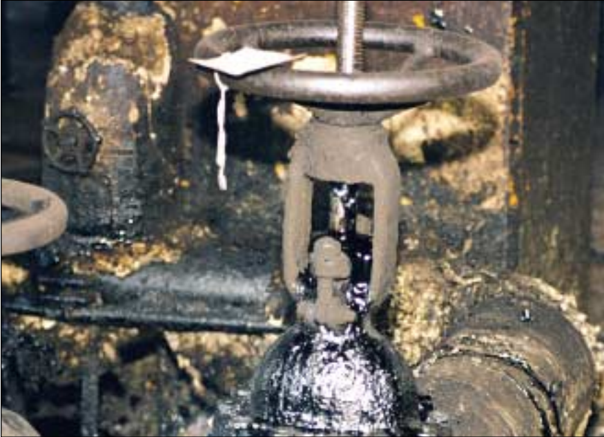
Photos shows contaminated valve in place tagged for cleaning.
